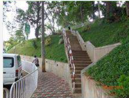
Construction of stair case and security post near main gate and renovation of pavement from main gate to Hanthana junction
