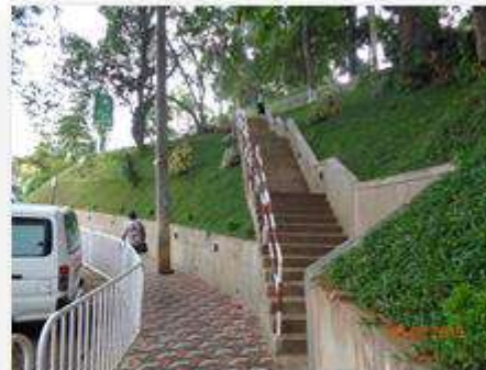
Construction of stair case and security post near main gate and renovation of pavement from main gate to Hanthana junction
